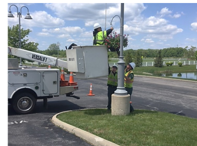
Crew members Rob, Shaun and Ian are hanging city flower baskets at the Public Service Department.
