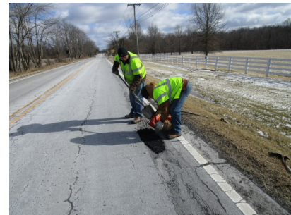
Filling potholes is not uncommon after low to high temperature swings.
