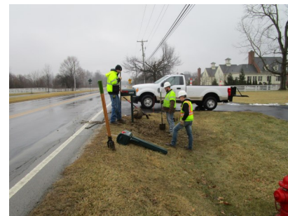
Mailboxes are sometimes damaged by the plow trucks during the winter months.
