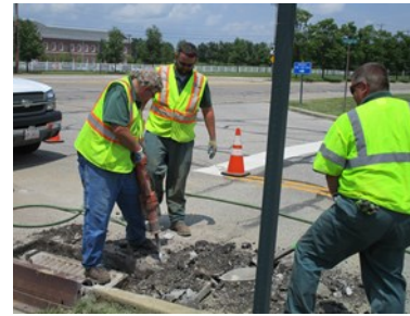
Crew members replacing the catch basin frame at Theisen Drive and US 62.
