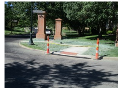
ADA curb ramps were improved at Lambton Park Road and Milton Court.
