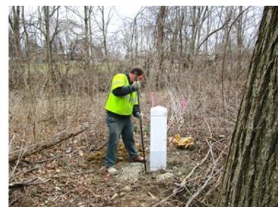
Service Worker Andrew Love installed corner posts at the New Albany Cemetery.
