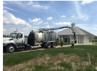
Service crews clean debris from sanitary service line at NA Parks Office.
