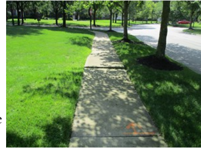
Typical sidewalk section to be replaced.
