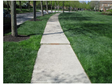
Typical sidewalk section to be replaced.
