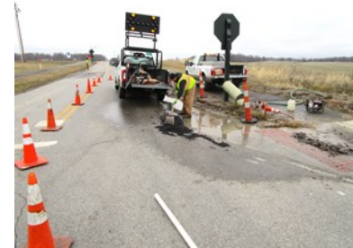
Pothole repair at the corner of Beech Road and Morse Road.
