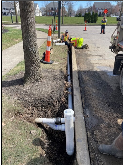
Maintenance workers Kerry Gastaldo and David Thatcher installed 30' of drainage pipe along Chatham Green Dr. Nick Sgandurra and Christian Duane managed the maintenance of local traffic throughout the area
