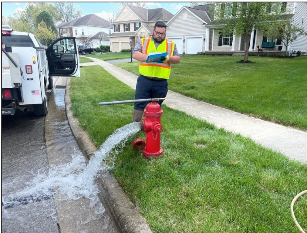
Maintenance worker Christian Duane performs hydrant flush while documenting the current condition of the hydrant on Marwithe Ct.
