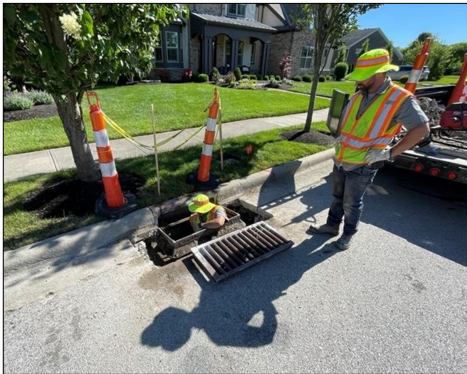
Nick Sgandurra and Kerry Gastaldo working on a concrete form installation in a curb inlet basin on McClellan Dr.
