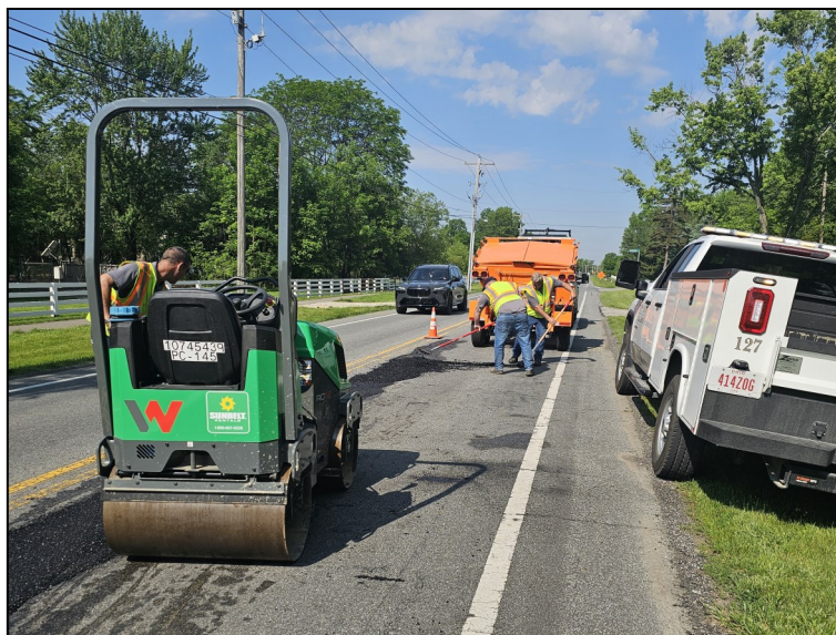
Keith Unterbrink, Chad Smith and Dennis Munsey placing patch and using the roller to seal patch job
