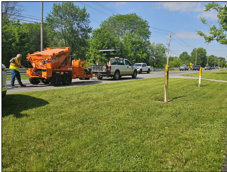
Dennis Munsey shoveling patch onto the roadway while Shaun Bush and Ian Hurst are flagging traffic
