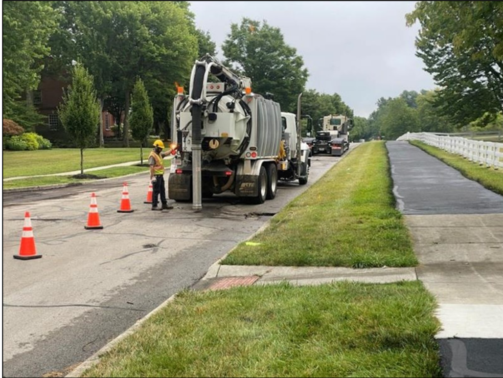
Nick Sgandurra performing a post-reconstruction cleaning of the storm sewer on James River Rd.
