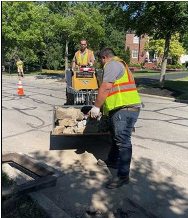
Nick Sgandurra and Christian Duane working on a catch basin frame replacement and structure reconstruction
