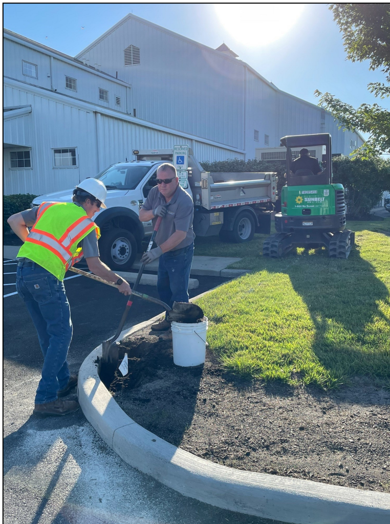
Tyler Myers and Mike Cligrow repairing irrigation and Steve Kidwell assisting on the mini excavator
