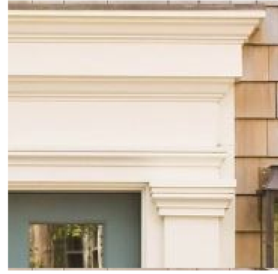
TR-1 material: trim and pediments manufacturer: tbd color: painted white to match FC-1
