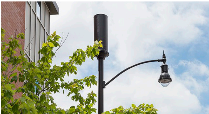
Example of a new small cell facility on an existing light pole.
