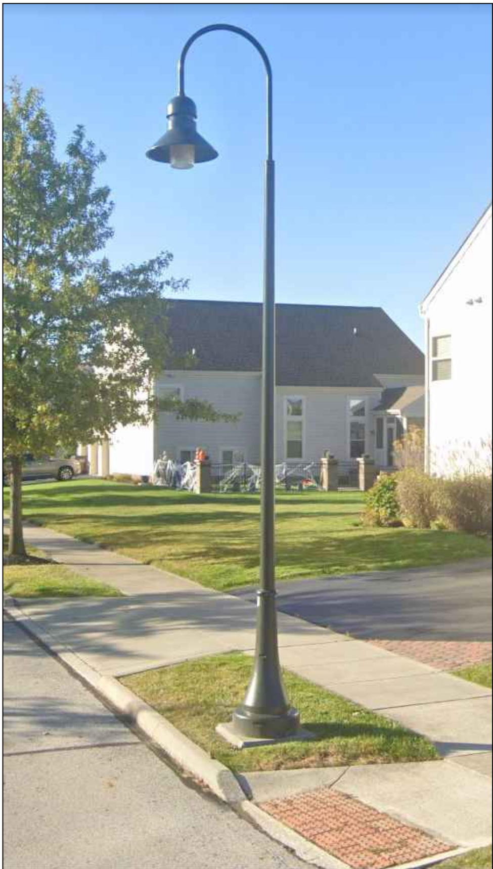
TYPICAL STREET LIGHT
