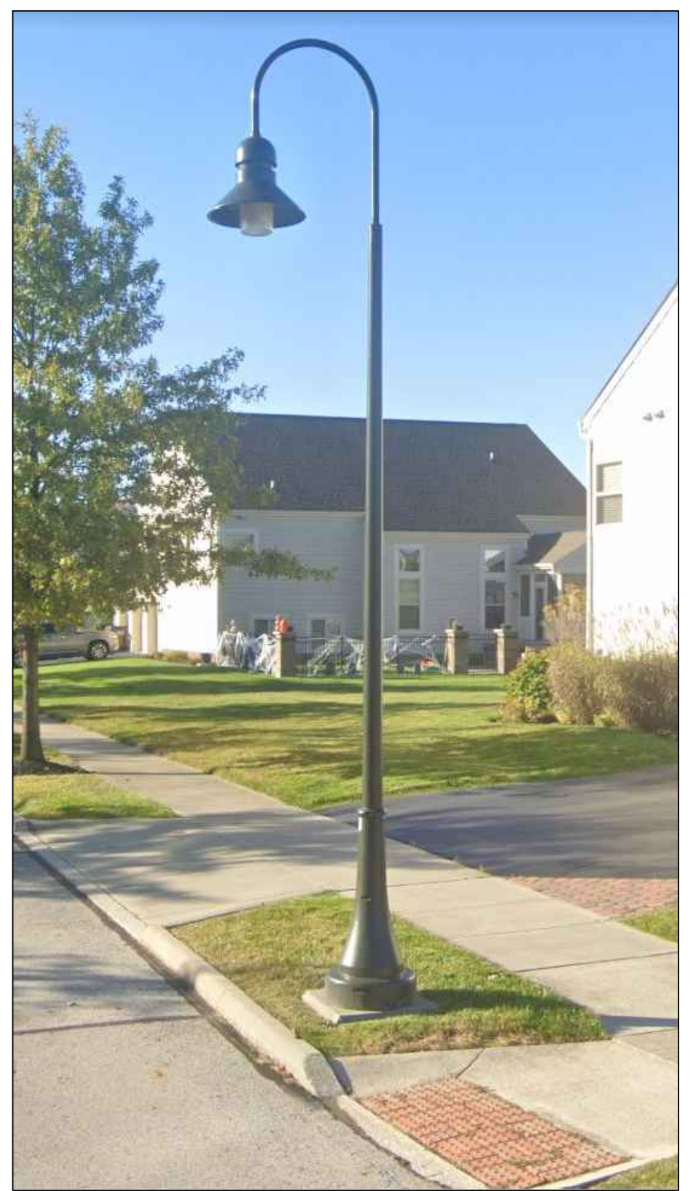
TYPICAL STREET LIGHT
